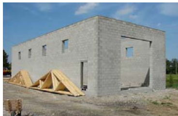
The new Road/Cemetery/Parks Dept. maintenance building takes shape at the Alkire Road facility.
