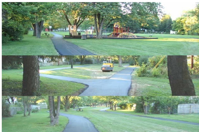
Three views of the walking path that was installed in Carl Frye Park this summer. The Road, Cemeteries & Parks Department laid out the path and put down the base. The paving was completed as part of the townships 2007 paving contract through the County Engineer's office.
